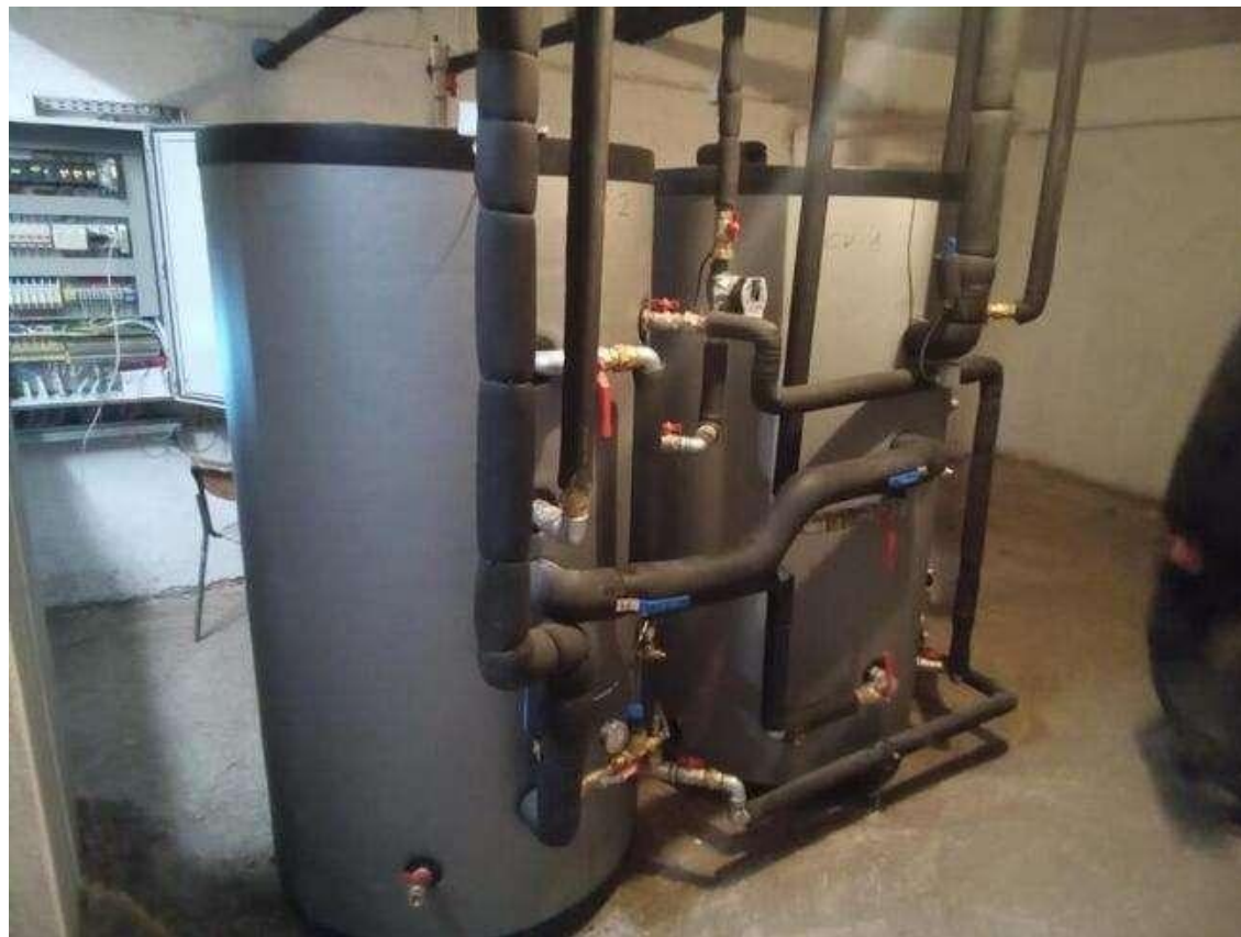
Domestic hot water tanks
