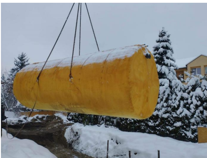
Underground heat storage tank 50 m 3 volume
