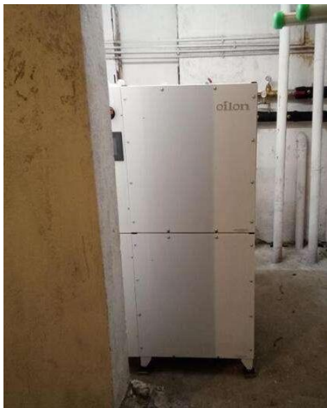
Heat pump Oilon RE56
