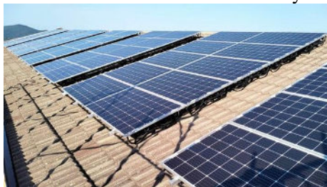
RESHeat system installation in Palombara Sabina
